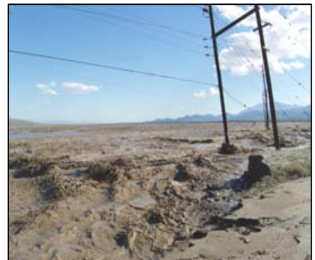
Flooding along Indian Canyon Drive, January 11, 2005.
