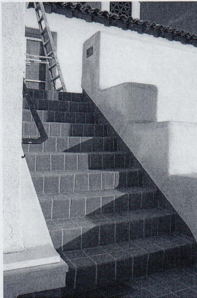
Stair decking to be replaced
