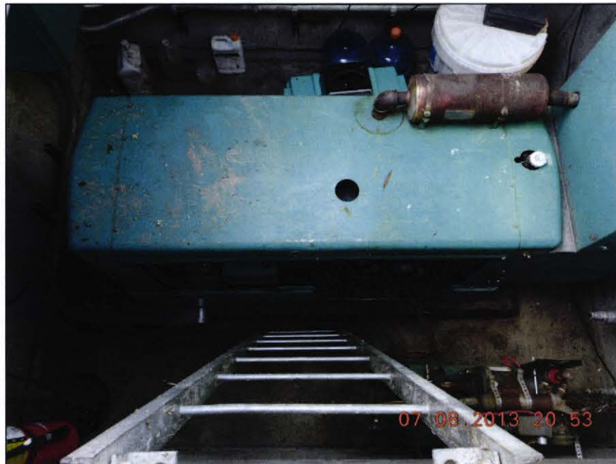
Photo of Emergency Generator at Lift Station No. 4
