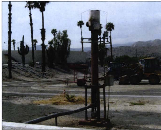
Photo of the Digester Gas Flare
