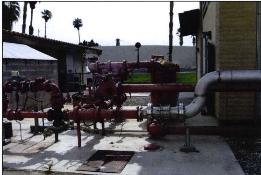
Photo of Anaerobic Digester Gas Flow Metering Section
