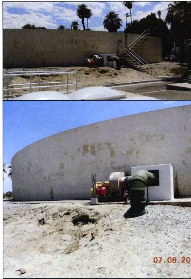
Photos of Slope Erosion Occurring near Trickling Filter #1
