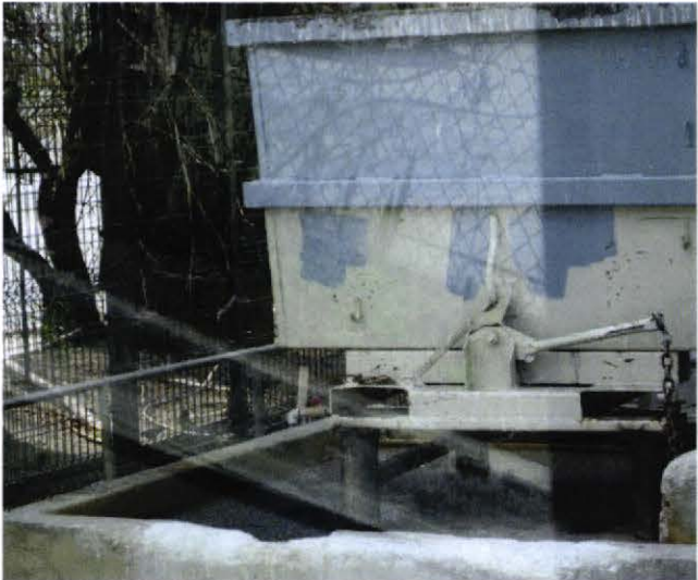
Photo of Damage to Concrete Containment
