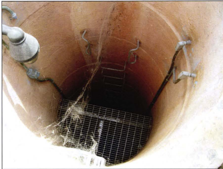
Photo of Lift Station No. 1 wet well coating damage
