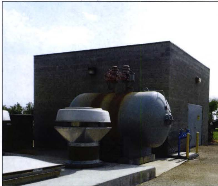
Photo of corrosion on hydro-pneumatic tank at Lift Station No. 1
