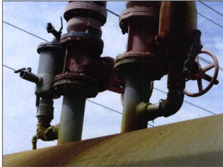
Photo of corrosion on hydro-pneumatic tank at Lift Station No. 1
