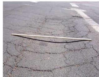
Rutting and Depressions
