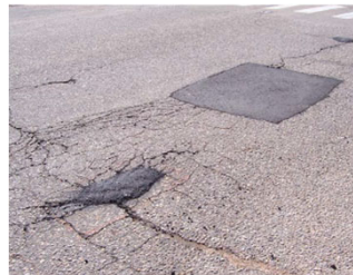
Patching and Utility Cuts
