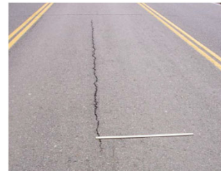
Longitudinal and Transverse Cracking
